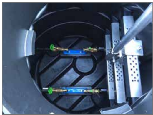
Water meter chamber with integrated installation fittings
