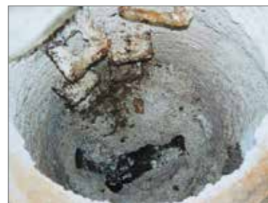
Starting point: corroded concret chamber
