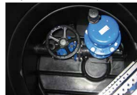
Venting- and exhaust manhole as side port
