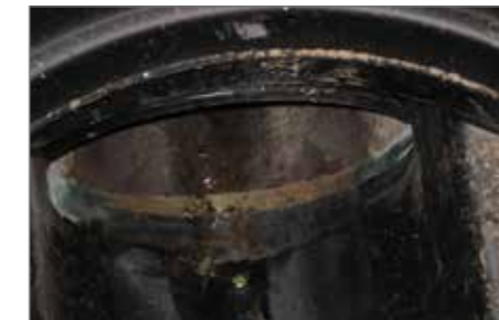
The PE pipe is connected to the old pipe using filling mortar
