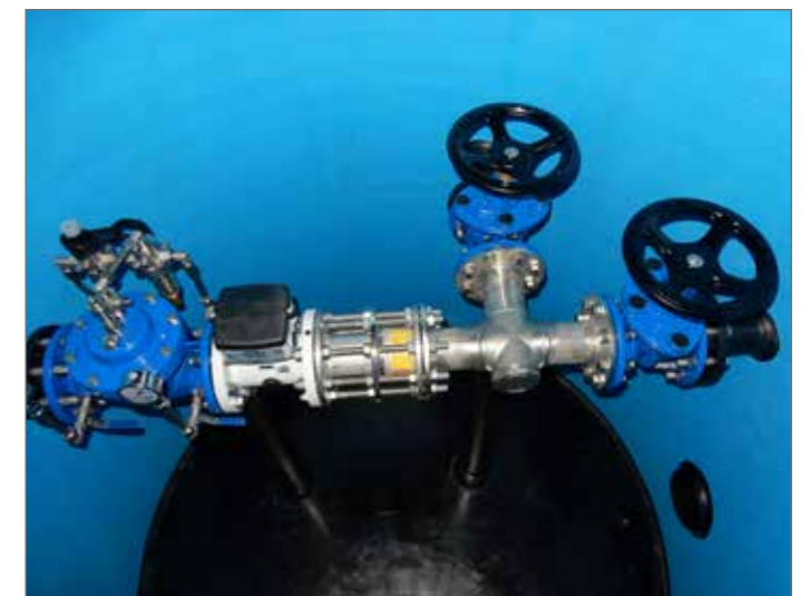
Distribution chamber with PE components
