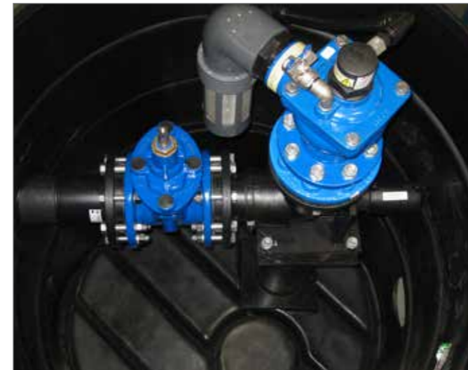
Ventilation and air release chamber with backflow protection
