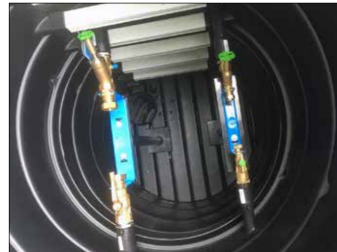
Distribution chamber with PE components
