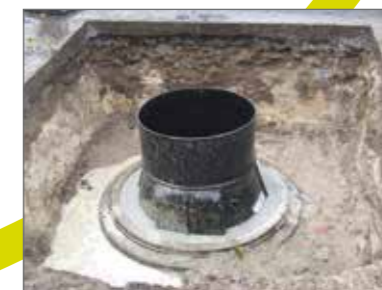
Filling the gap between DN 800 PE chamber and DN 1000 concrete man- hole with filling mortar
