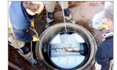
5.) Adapt the prefabricated channel with PE socket and place it in the chamber bottom
