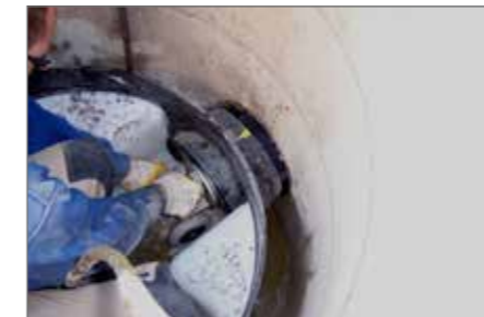
6.) Set the sealing plug for the inlet and outlets, fill the gap with modified filling mortar
