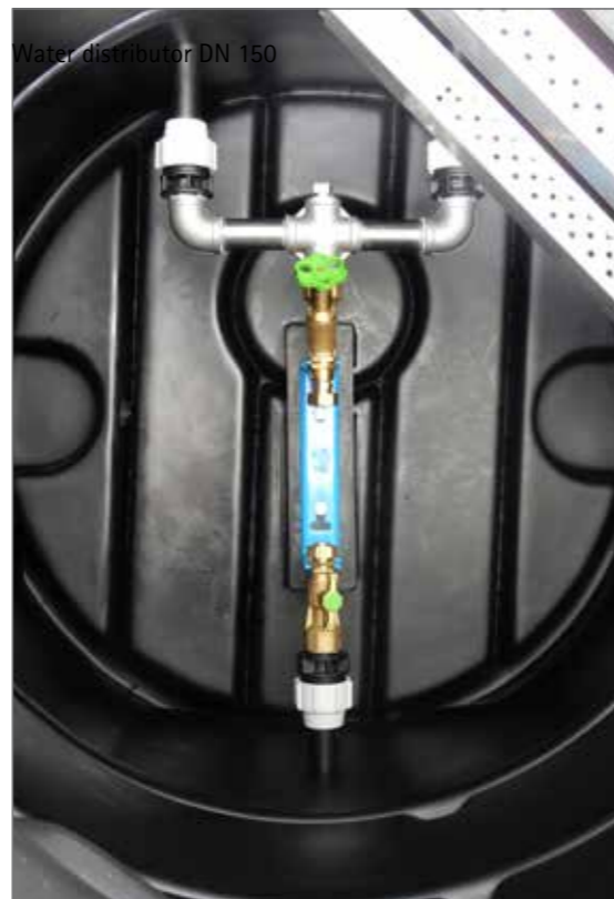
Water meter with downstream distributor
