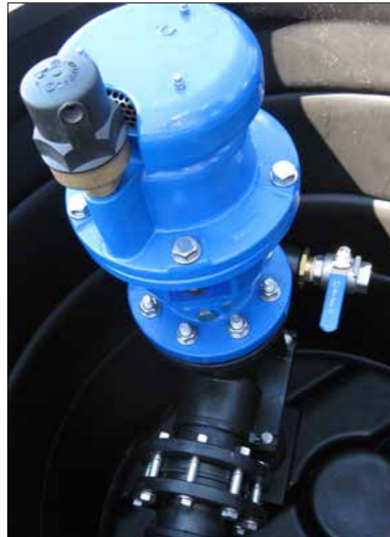
Distribution chamber with stainless steel components
