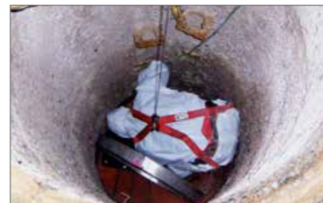
3.) Cut the asphalt, and lift out the concrete cone and remove steps
