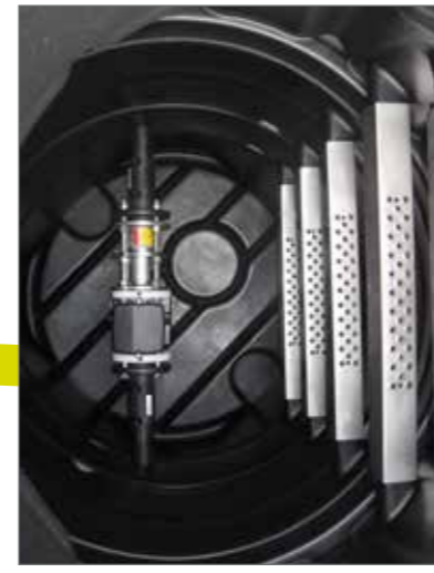
Water meter chamber with MID-measure
