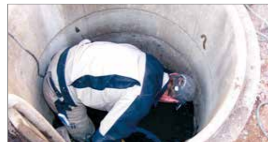
2.) Remove climbing steps, reduce berm and flume, water retention, set the over-pumping operation
