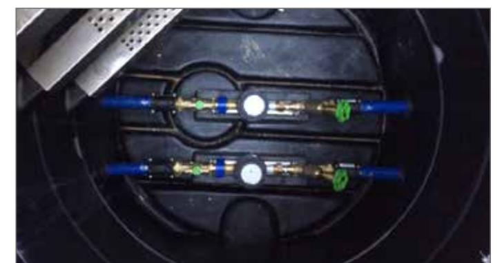
Double water meter chamber
