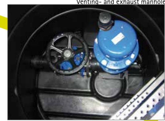
Venting- and exhaust manhole
