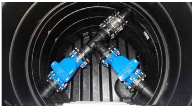
Junction valve with manometer
